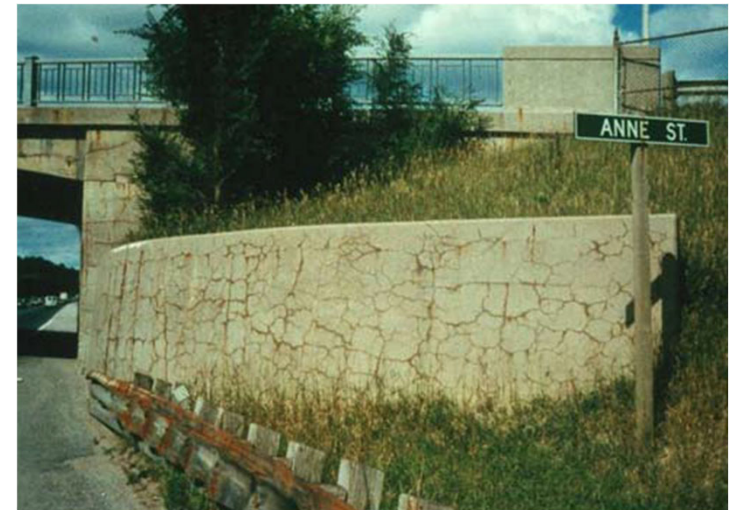
the pathology observed on site
